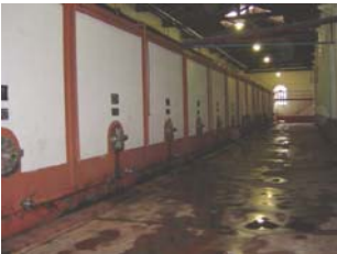
Epoxy lined chambers...
